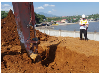
Sampling shore stockpiles
